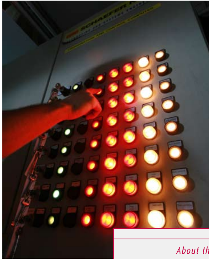
The control system/sensor board of YCH's ASRS system.
